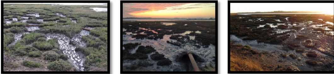
Channel system, after the installation of coir logs, during and after completion of pumping operation.
