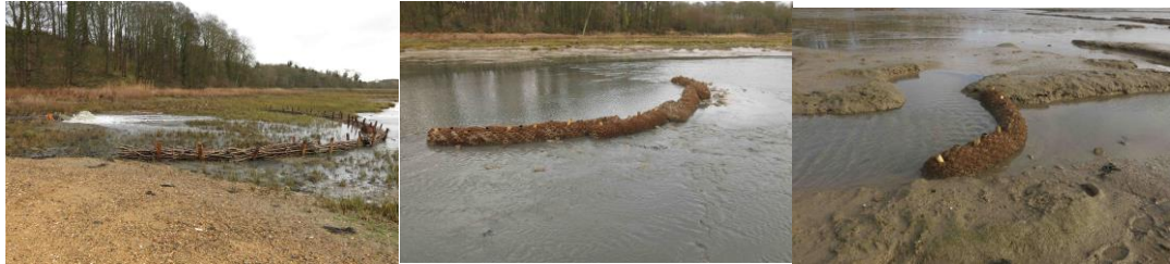
Holding pen at discharge point Coir bund at upper channel Single coir log in small channel
